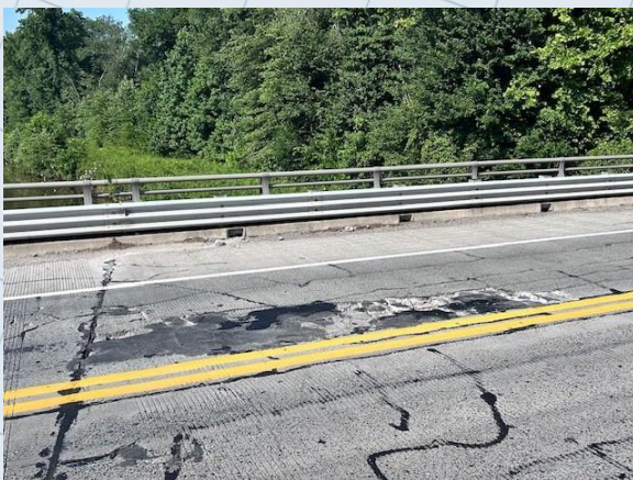
View of Concrete Delamination and Spalls in EB Lane
