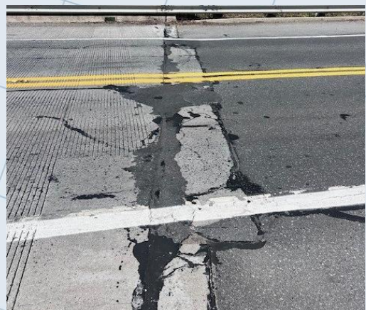
View of Spalls filled with Cold Patch Asphalt on the West Approach
